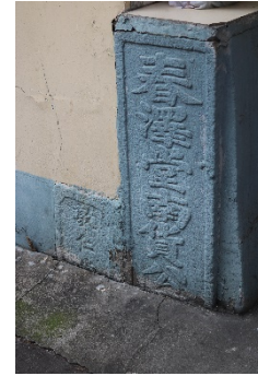
Fig.4. Chunze Hall south goods public sector monument (Source: Taken by the author on January 1, 2020)
