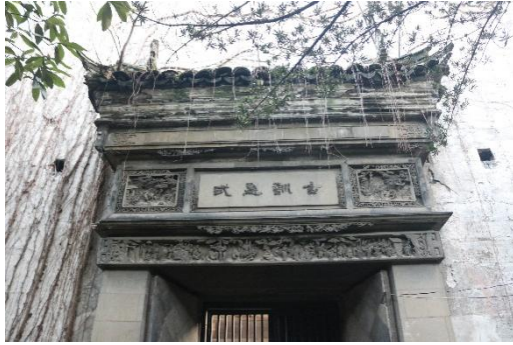
Fig.3. Brick carvings gates of the hidden building (Source: Taken by the author on January 1, 2020)
